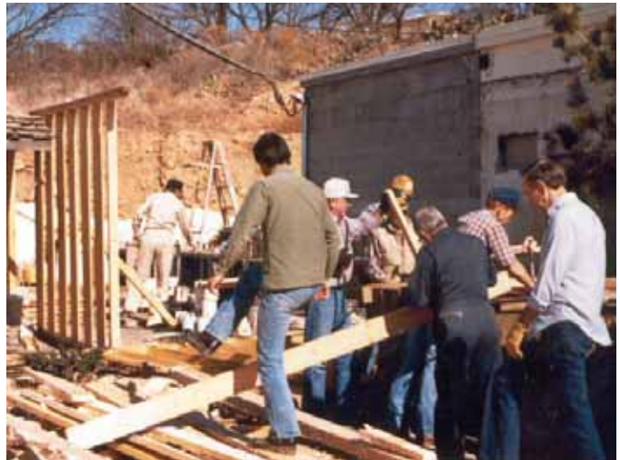
Squadron members tear down a storage building at the Ridge Restaurant for materials (1985)
